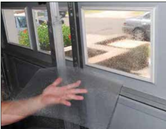
Fig 4-21. Laminated film comes in various thicknesses and strengths. Here the film is applied to an existing window before it is fastened to the frame with silicone structural sealant.
